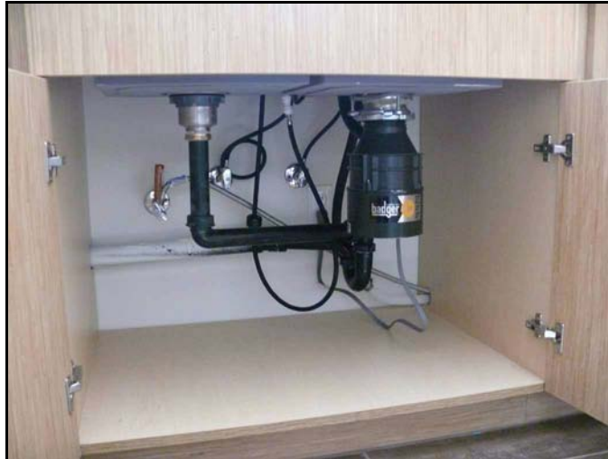
Garbage Disposal Under Kitchen Sink
