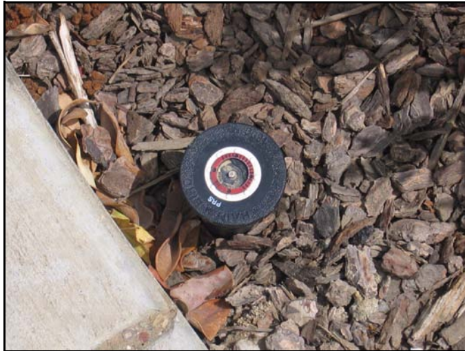
Irrigation Sprinkler Head
