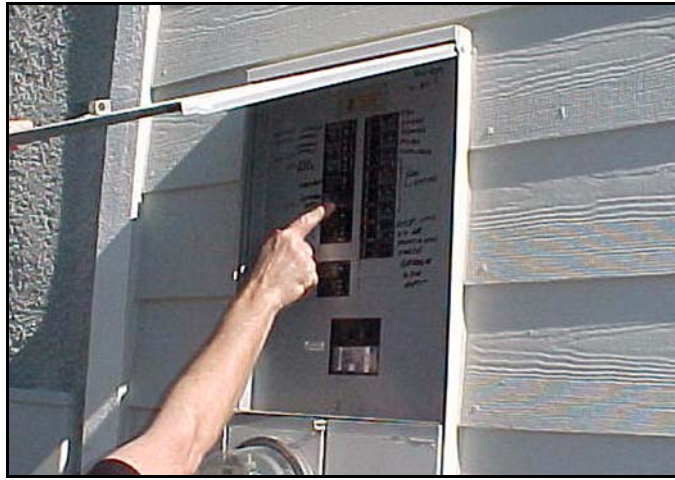
Exterior Circuit Breaker Panel
