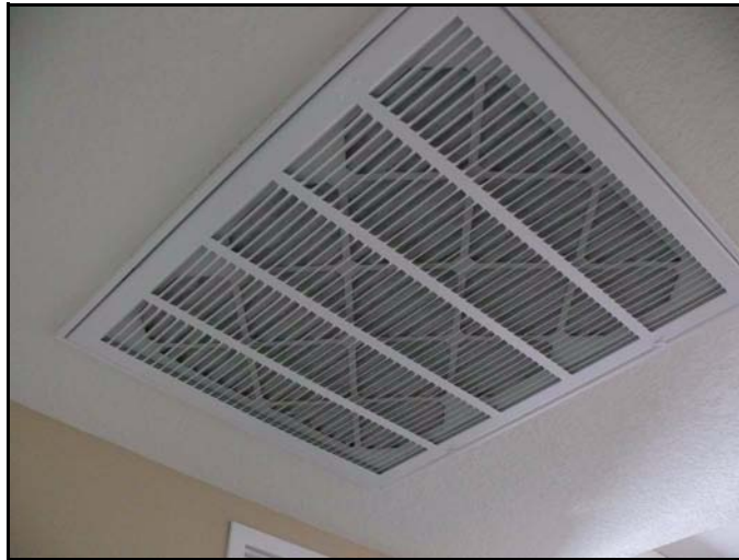
Example of an Air Filter Location
