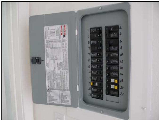
Interior Circuit Breaker Panel
