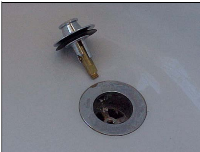
Drain Trap in a Bathroom Sink
